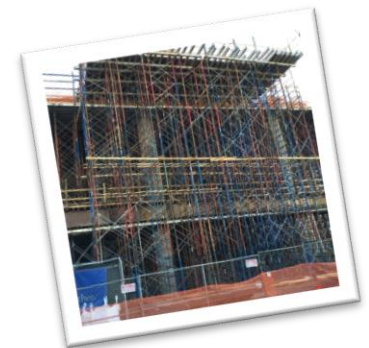
What is with all that wood? The wood, also known as shoring, provides support until the structure is complete.
