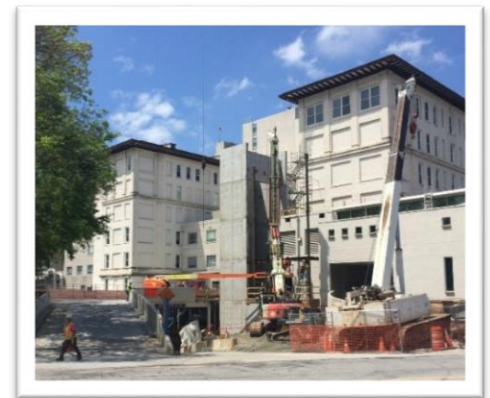
Installation of the steel structure for the bridge supports has begun on the main hospital.
